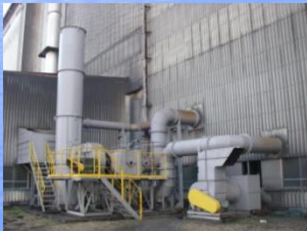
NYB Outdoor Exhaust Facility 3 years after construction
