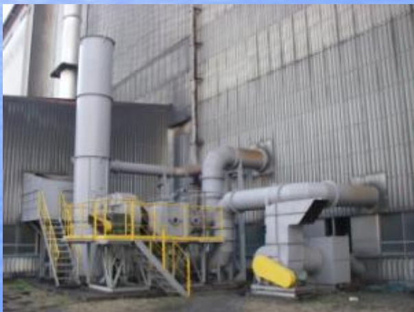
NYB Outdoor Exhaust Facility 3 years after construction
