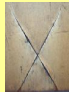
SlagLead SR 3 deterioration
