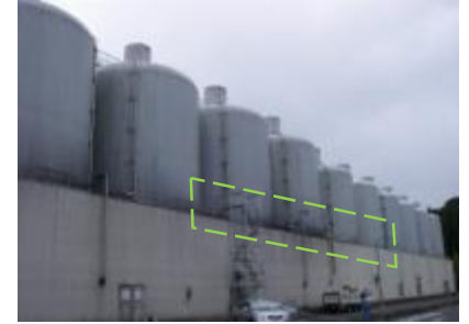
Base of beverage tank
