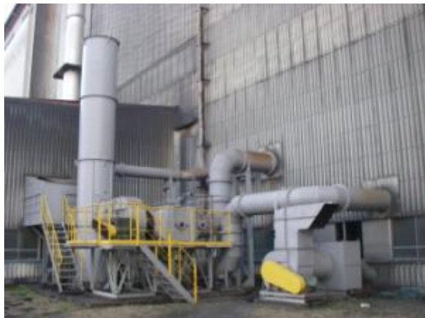
NYB outdoor exhaust equipment 3 years after construction
